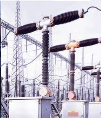
CORONA, PARTIAL DISCHARGE DETECTION
